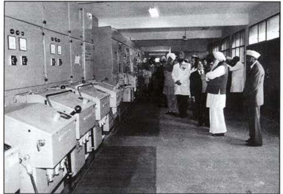
The hospital's electrical substation.
