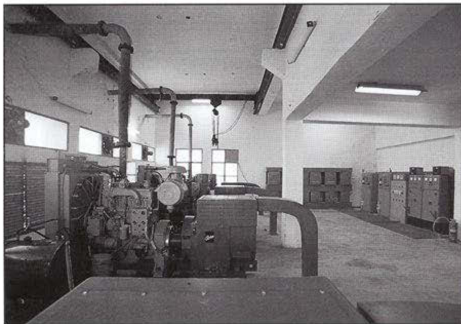
Diesel emergency power-supply generators.
