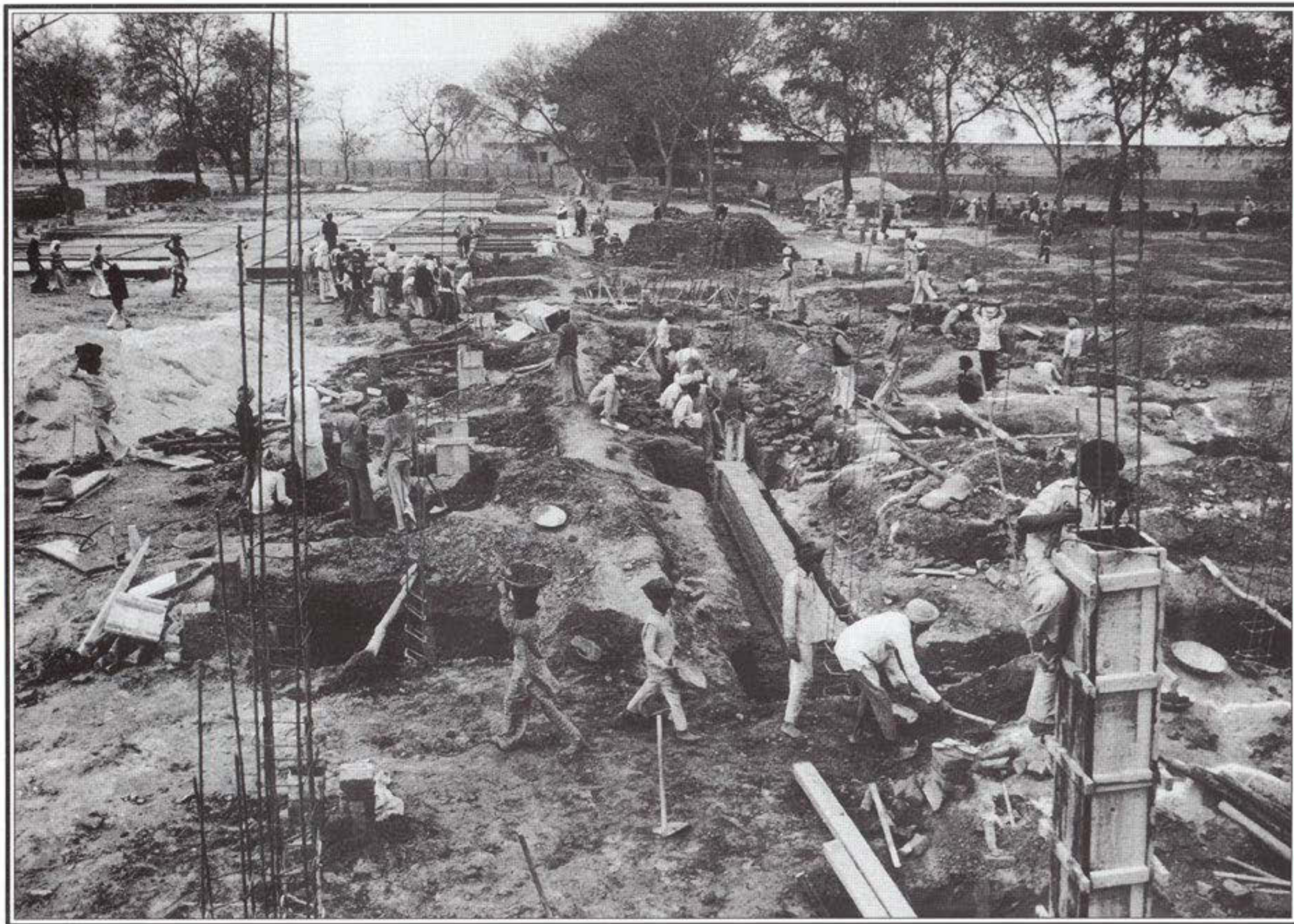
Digging foundation trenches at the hospital site during the early days of construction.
